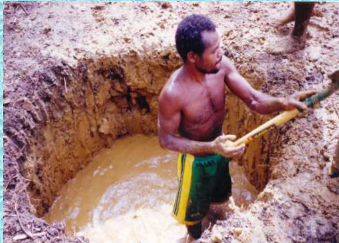
A shallow well is dug by hand and is limited to 7 m depth. It is less expensive and can be constructed anywhere. Water can be pumped or bailed to the surface with bucket and rope.
