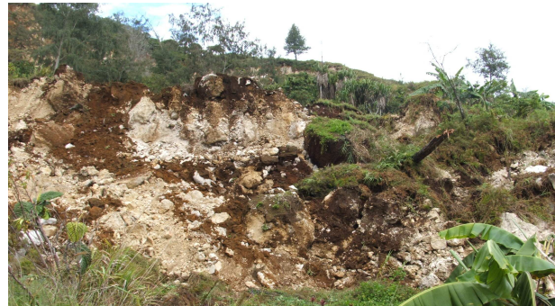
Landslide at Wamai, Highlands Highway, Chimbu Province
